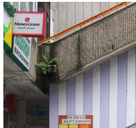
Fig. 5. Fern development on the Cluj-Napoca building wall, August, 2011
